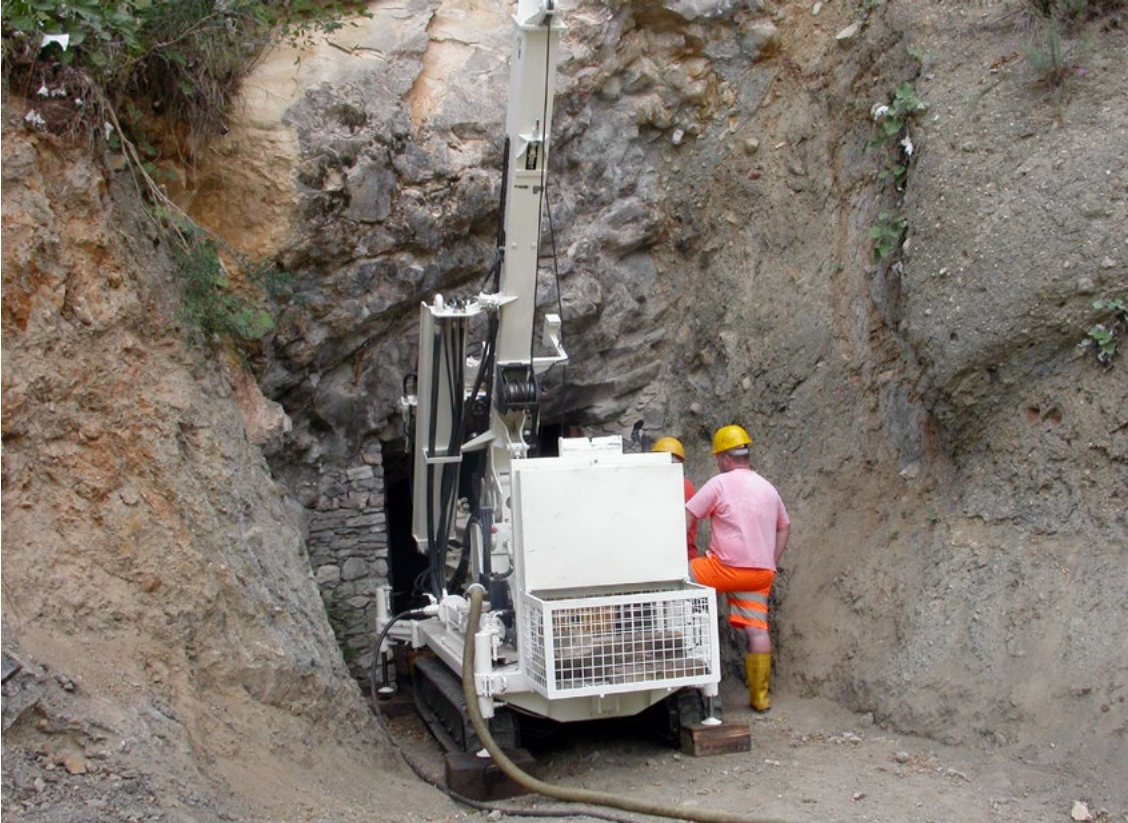
Pesciara: continuous core sampling carried out in 2011 in correspondence with the lower tunnel where there is contact between Eocene limestones and volcaniclastic rocks
